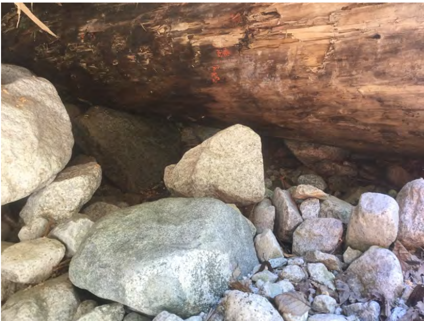
Downstream left sill scour
